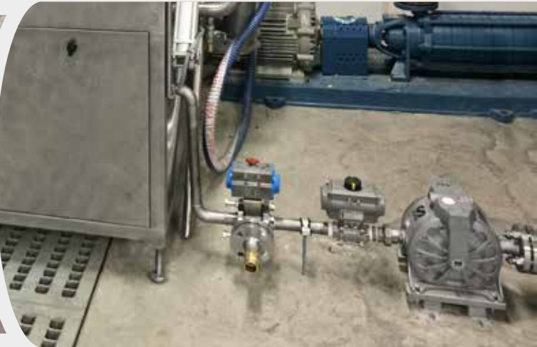
Chemical products dosing.
